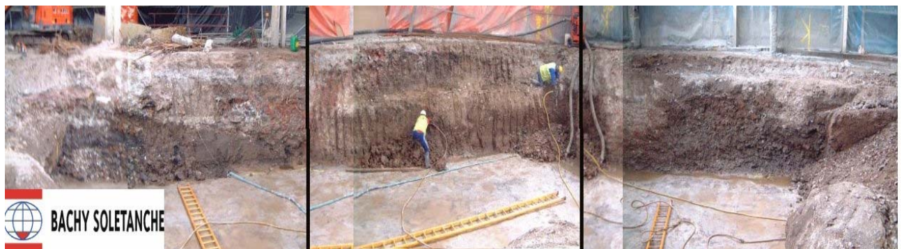
Exploded View of North, East and West Faces of Jet Grouted Wall After Excavation Providing Gravity Excavation Support Without
