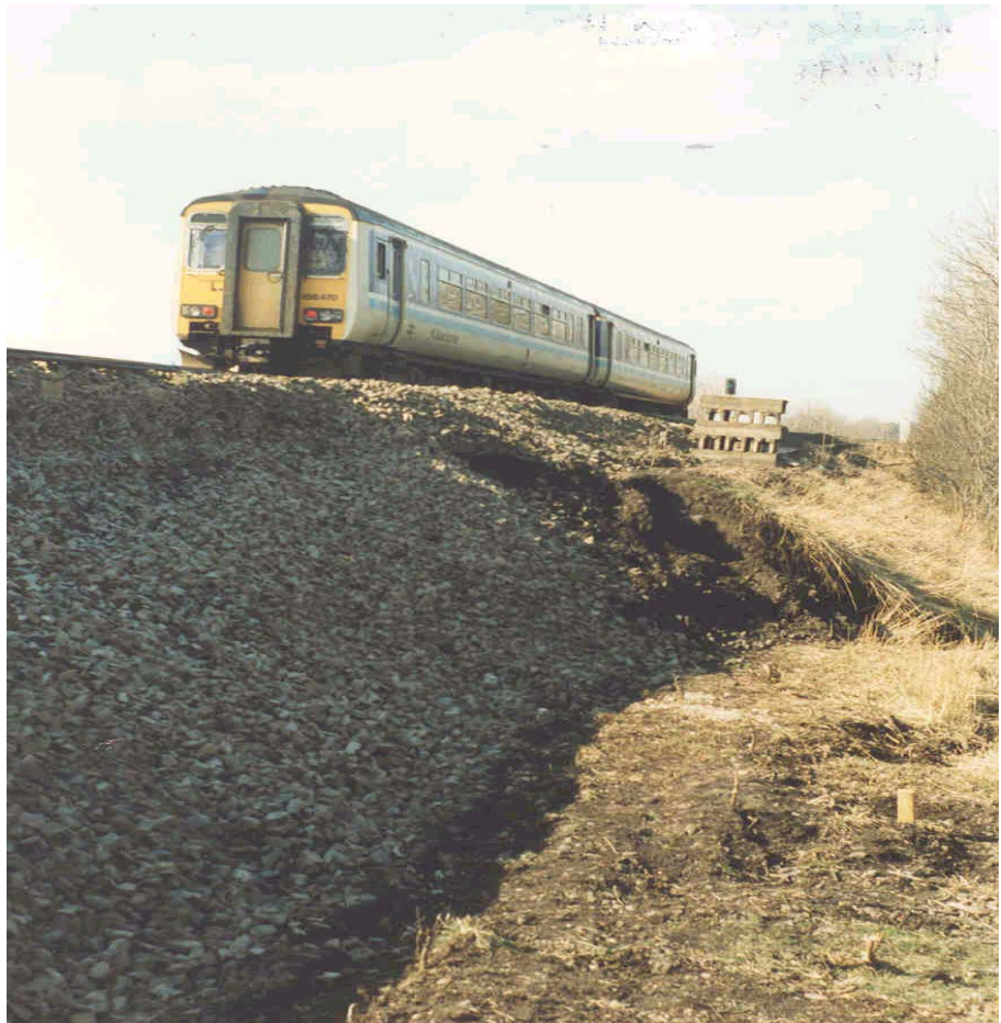
Site of major slip failure prior to commencement of remedial work
