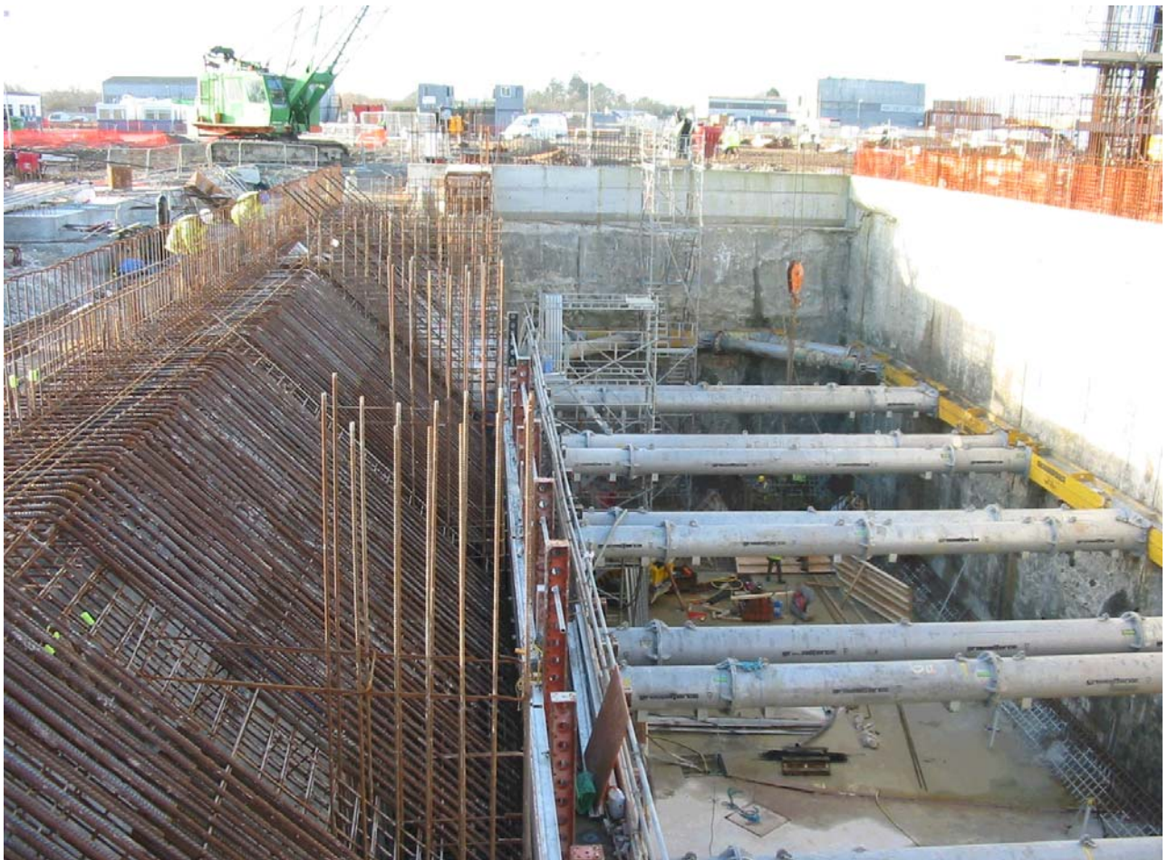
Bunker Structure - Tipping ramp construction in progress / propping installed with bottom up dividing wall in progress
