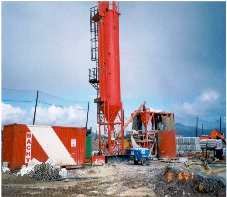
BSL mixing plant area
