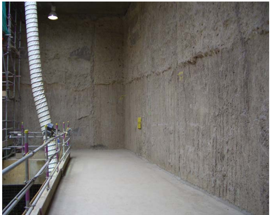
The above photograph shows the exposed wall. The difference in the texture of the surface of the wall is due to the ground strata. The top half of the wall was excavated through sand and gravels but below the visible line the ground was made of stiff clay.
