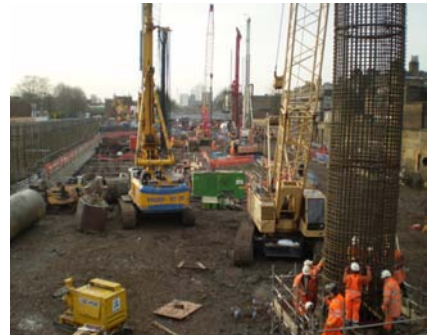
Dalston Junction Station piling including installation of a reinforcement cage for 2100mm dia piles
