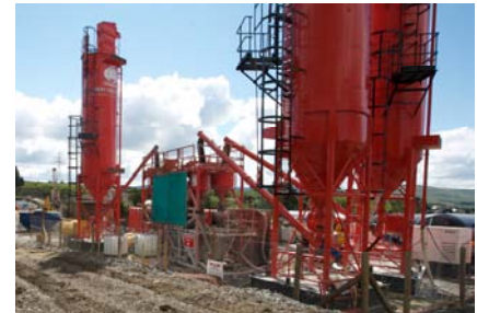
On-site Slurry Mixing Plant
